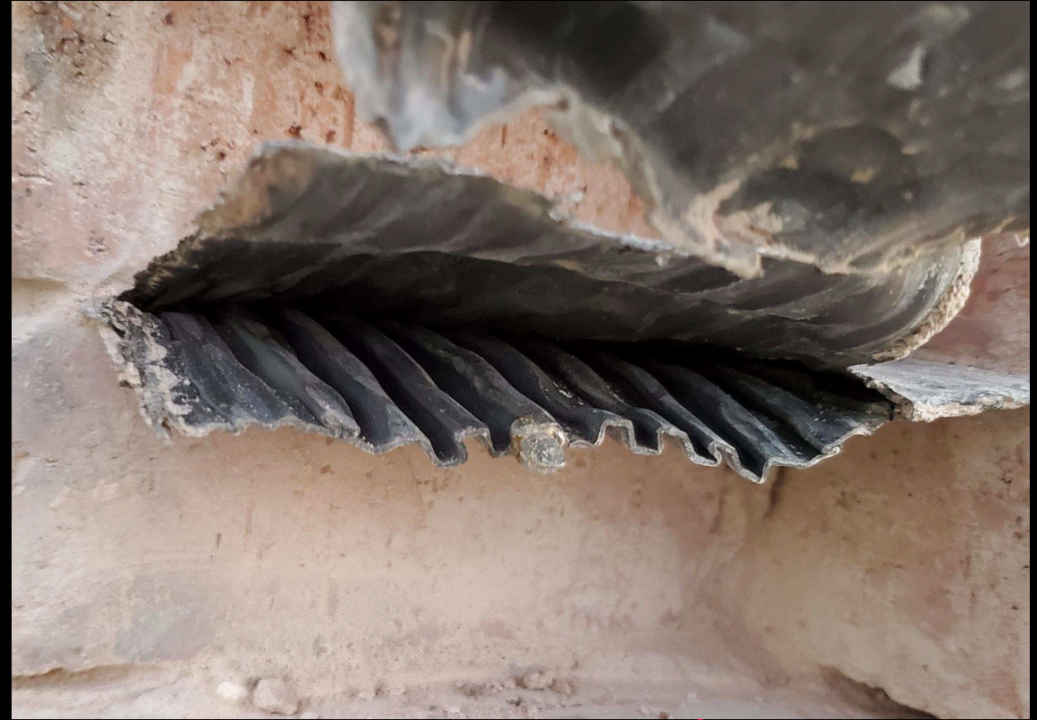
Peeled Back Expansion Joint Material
