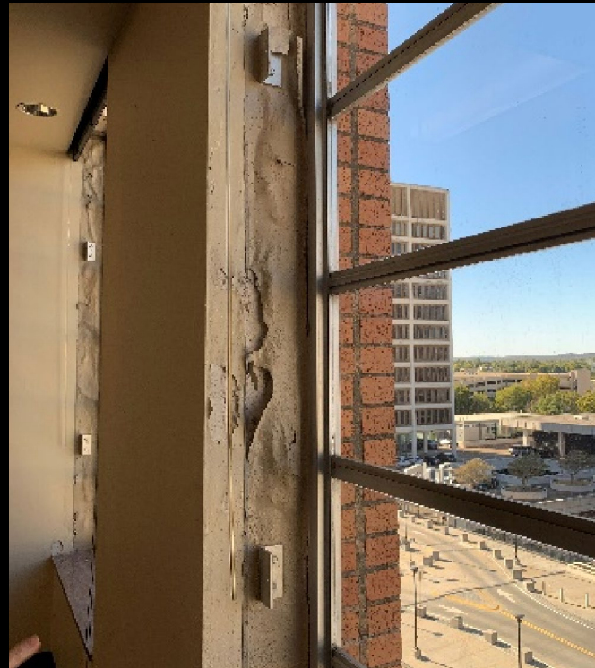
Water Damage Photos
